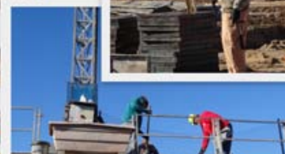
Pictured above is Shane Hale and Steve McCain at Marion Highschool working for Wagner Masonry.
